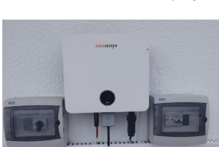
Location: Tunisia Capacity: 3kW
