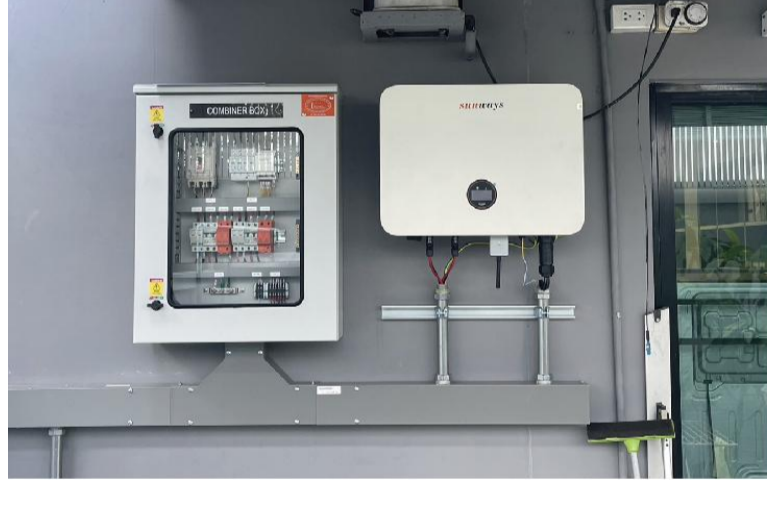
Location: Thailand Capacity: 10kW
