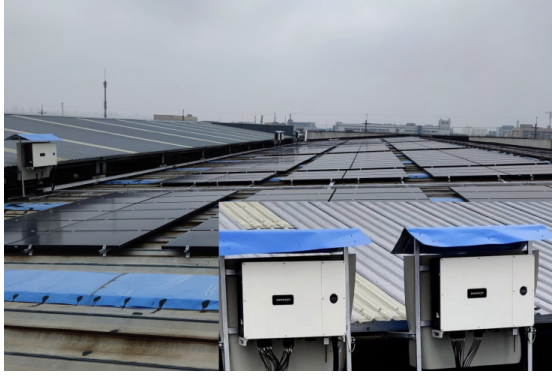
China 400kW Commercial Project
